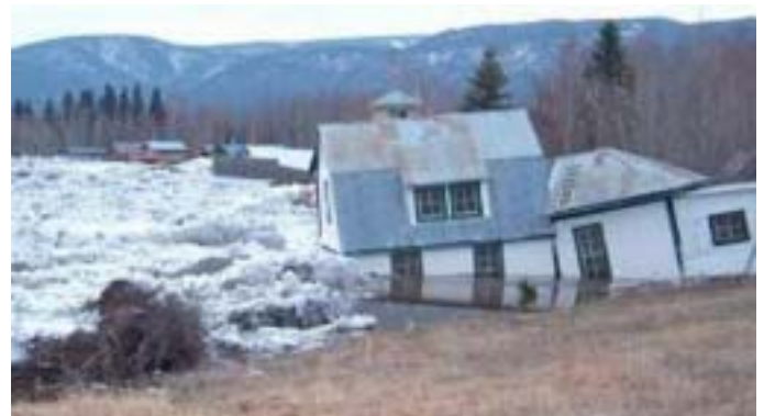
Below: Water and massive ice chunks flooded the town of Eagle, destroying this home in May, 2009.
