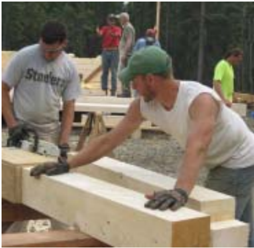
Mike Mock (left) works a chain saw while Jordan Speigle steadies the lumber as they help reconstruct one of the new homes in Eagle, Alaska
